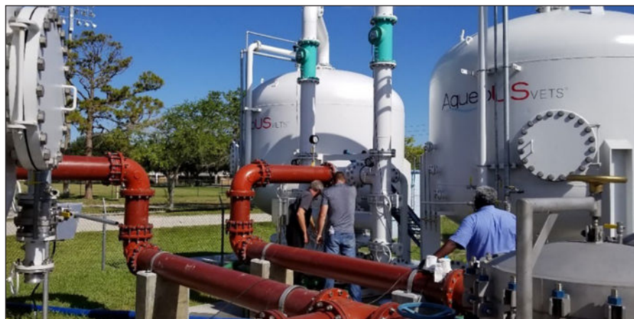
Figure 11. Start-up of the system.
